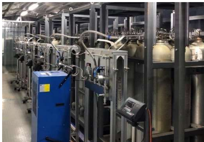
Gas storage system
