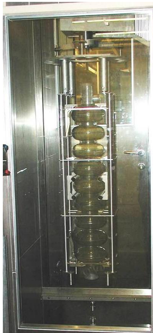
Rinsing cabinet of "new" DESY HPR system with "plastic" cavity
