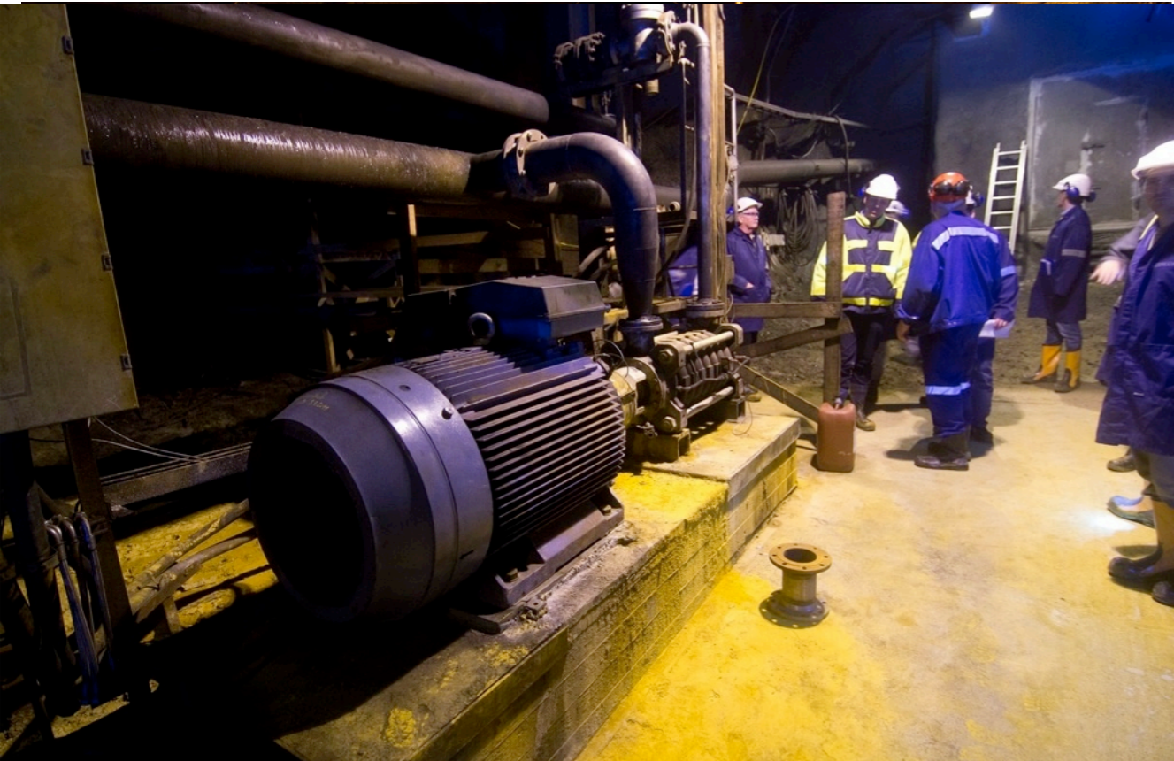
This pump alone takes all the water from 645 m to the surface
