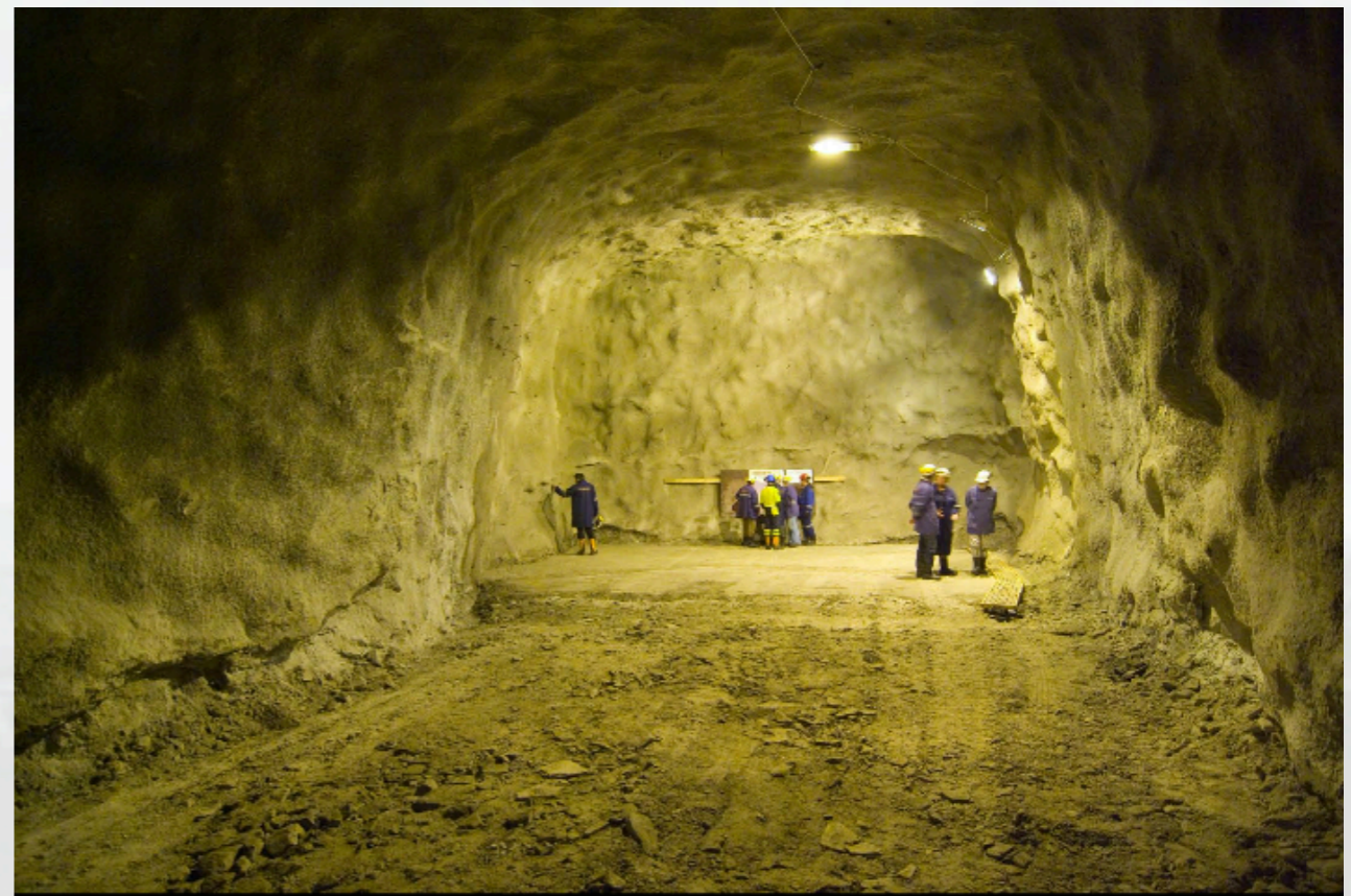
250 m long tunnel and a cavern at 1400m excavated for LAGUNA R&D
