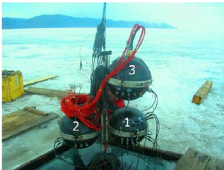
Fig. 10. FADC sphere (1), String PC unit (2), and LED flasher sphere (3) after final installation
