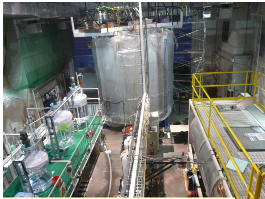
Liquid hall: LS production and filling
