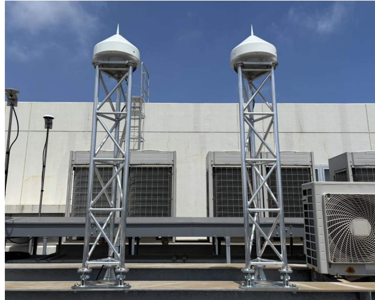
GNSS Antenna installed at JPARC Neutrino building
