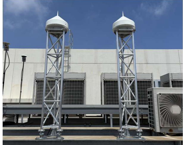
GNSS Antenna installed at JPARC Neutrino building
