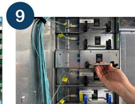
9 The drive is now considered a Spectra Logic certified drive and is covered by the same Spectra support contract as all other drives in the Spectra Cube and is now ready to be used in production
