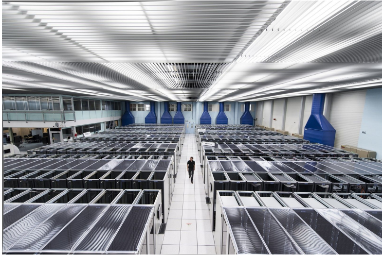
CERN Data Centre
