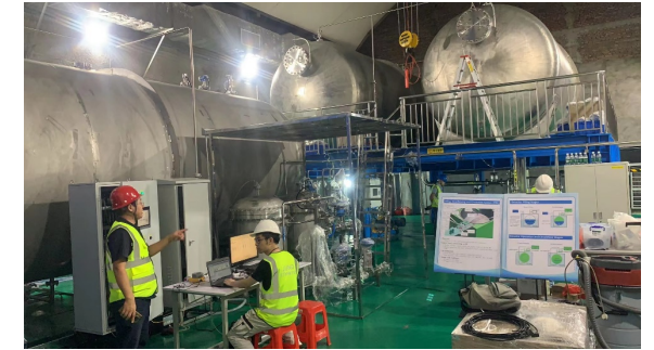
Filling Overflow Circulating room
