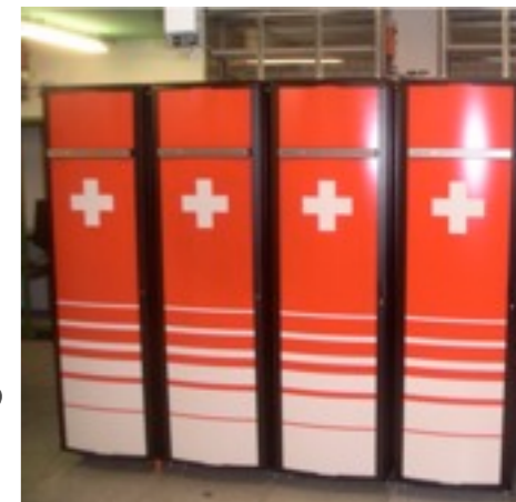
Source: ETH CSCS
