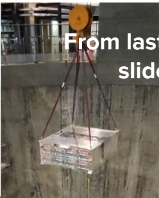
HA-TPC installation (Sep. 2023)
