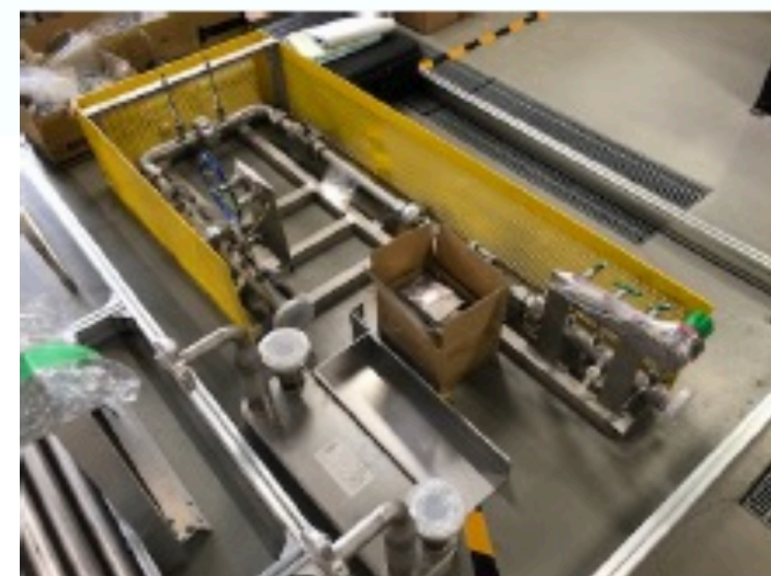
New target cooling system
