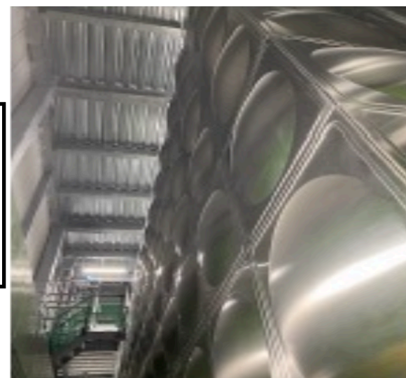
New water tank for radioactive water disposal
