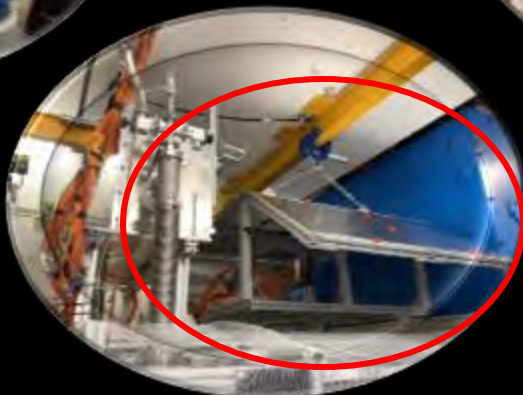
VELO-TOP NTD array installed
