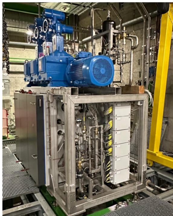
Major progress with CO 2 cooling plant for ITk & HGTD Infrastructure installed at P1
