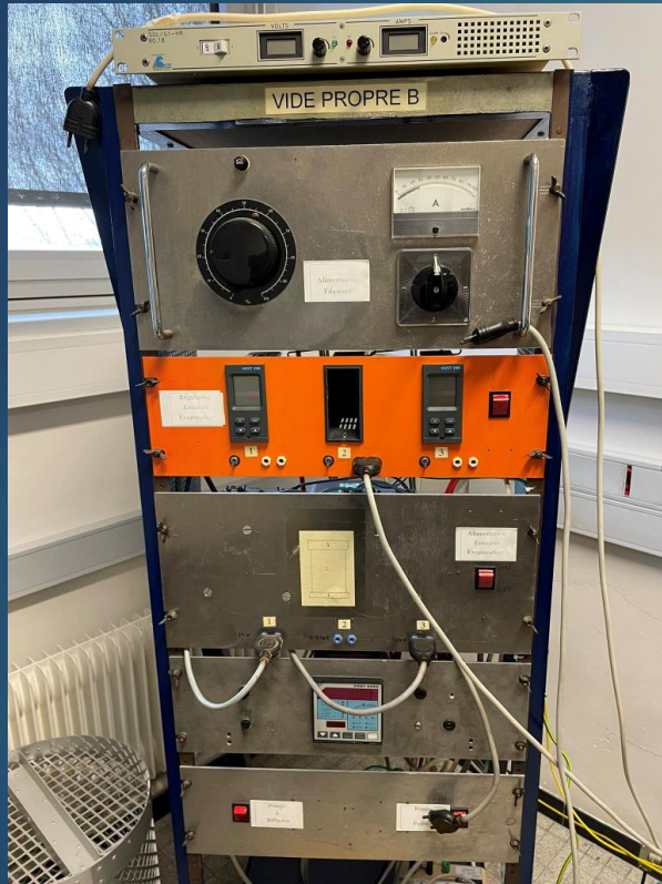
Central control panel (pumps + thermocouple)
