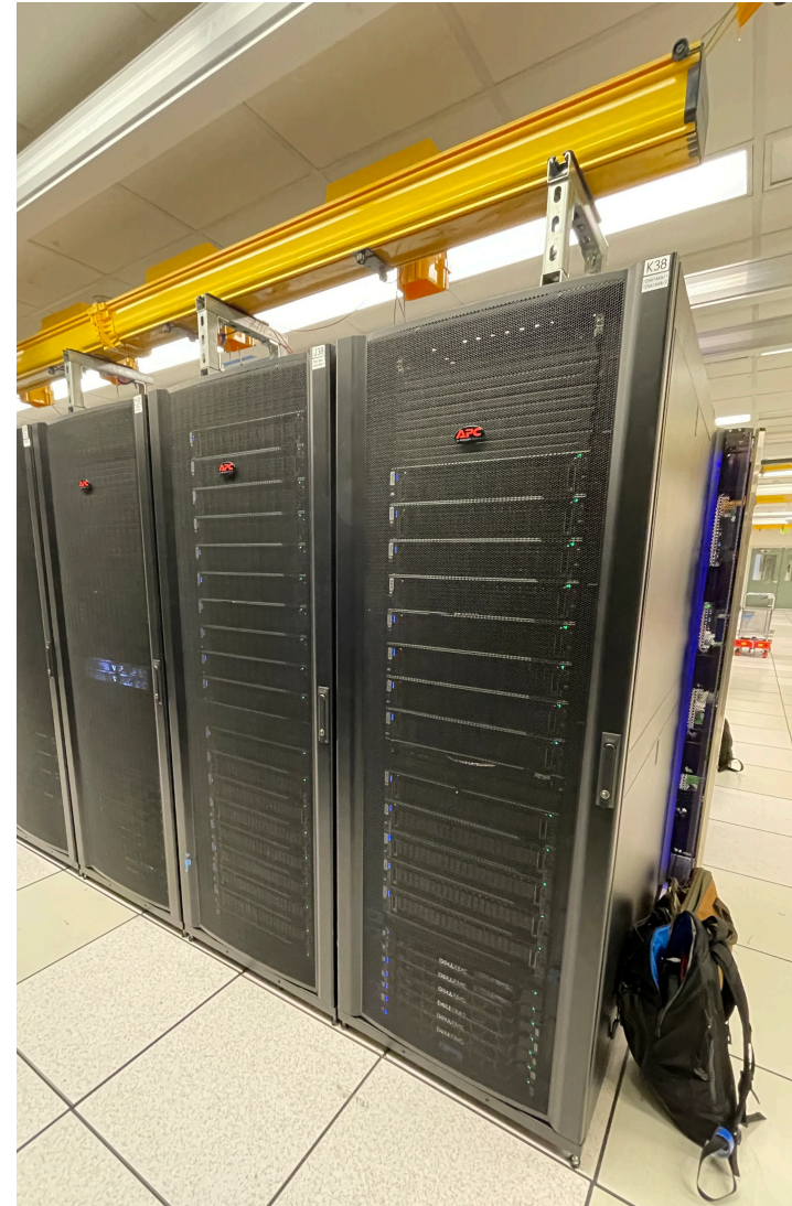
Cluster Racks in 50B-1275 Data Center
