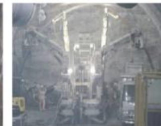
Erector/ Spray Machine
