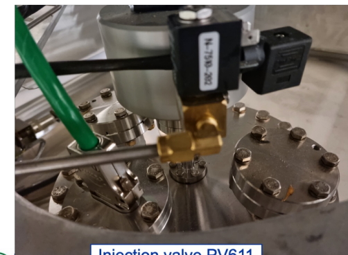
Injection valve PV611
