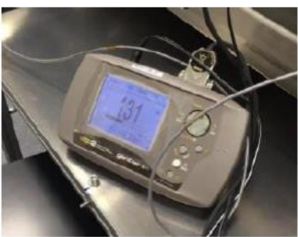
Installed and tested on Virgo
