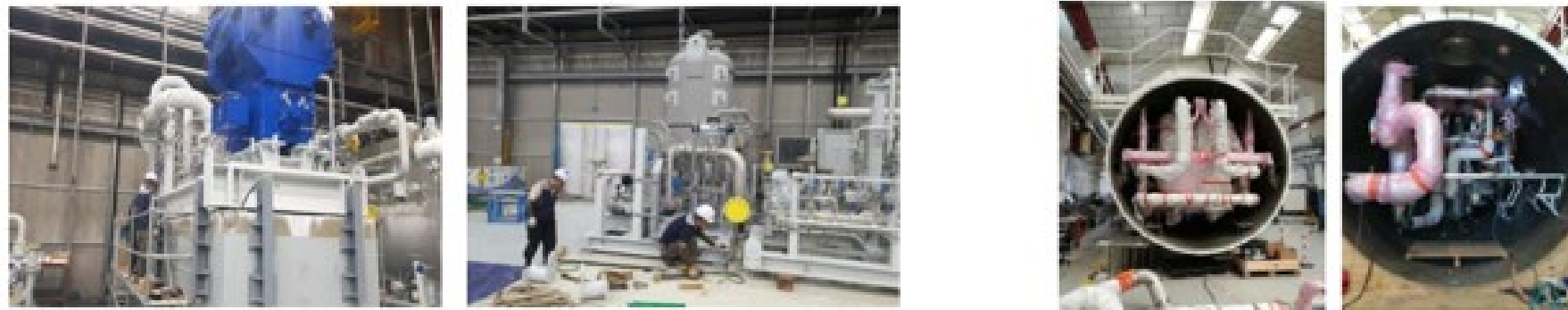
Compressors and Oil Removal System (WCS)
