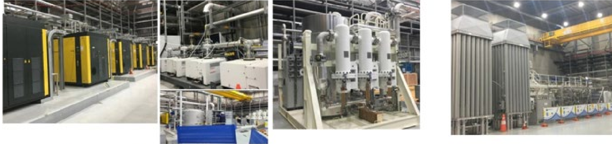
Compressors and Oil Removal System (WCS)
