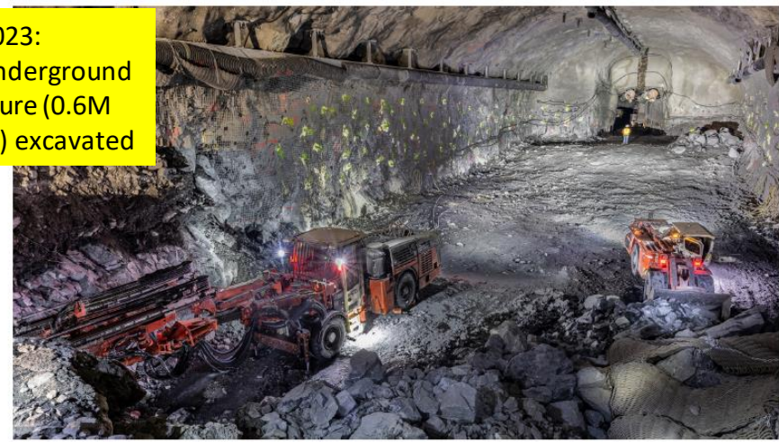
Drilling holes for blast charges for bench C (left) and removing muck (right) in North Detector Cavern (4850-33)
