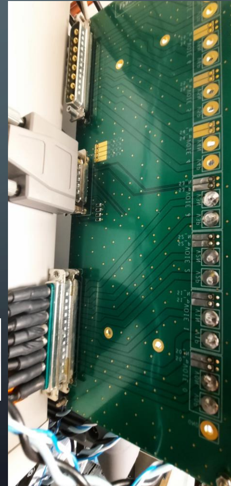
Channel 0 is power on for several weeks
