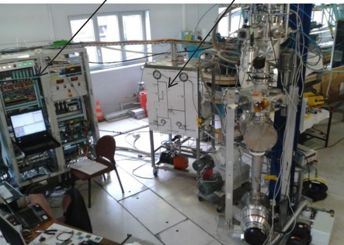
Instrumentation rack Transfert GH2 rack
