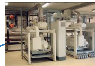
He pumping station for the cryo test hall
