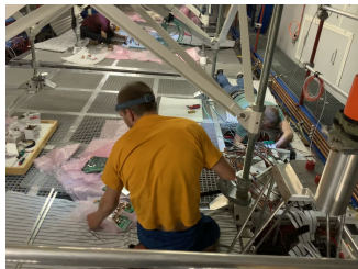
Figure 6: Installation on the MTPCs
