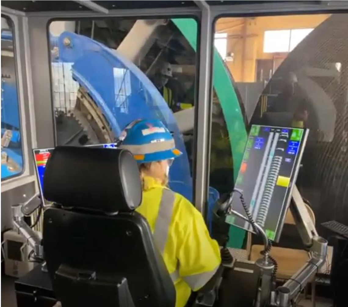
Operator Hoist Control Center with Flat Screen Monitors and Joystick Controls
