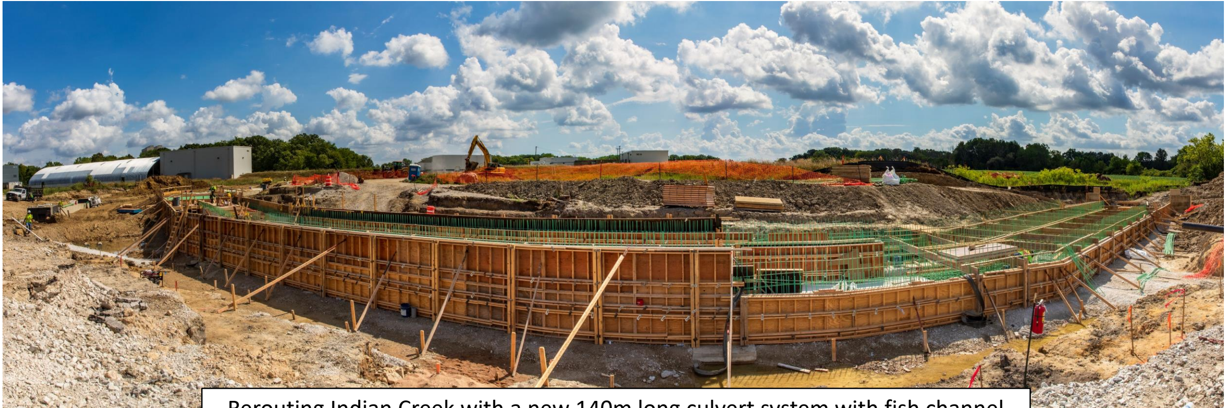
Rerouting Indian Creek with a new 140m long culvert system with fish channel
