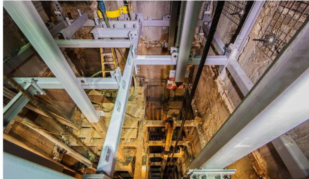
Renovation of Ross Shaft in progress, with old and new structural steel sets visible.
