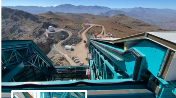
Shutter Seals (view towards AuxTel)
