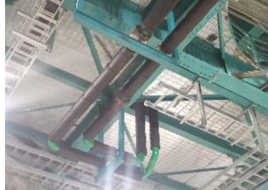
Oil piping level 5
