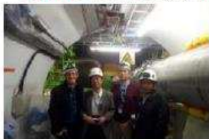
LHC beam dump
