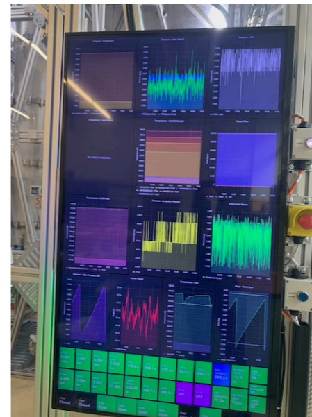
Slow control screen in the operations room
