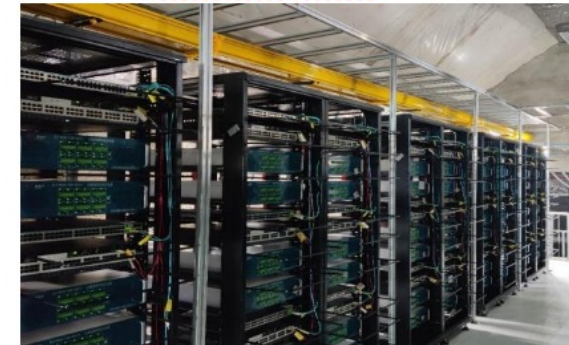
underground electronics room
