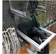
(c) Optical fibers at patch-panel
