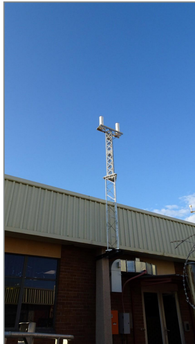
First installation in South Africa
