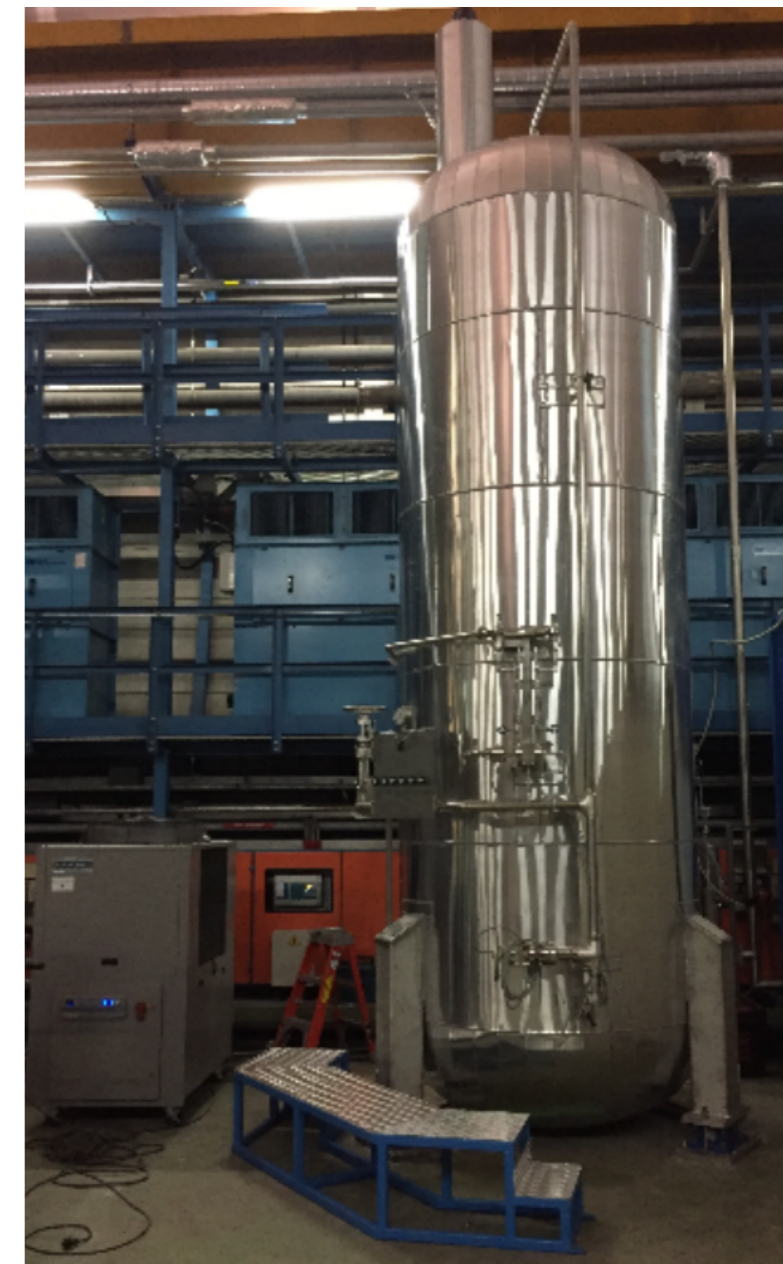
ReStoX2 installed in LNGS
