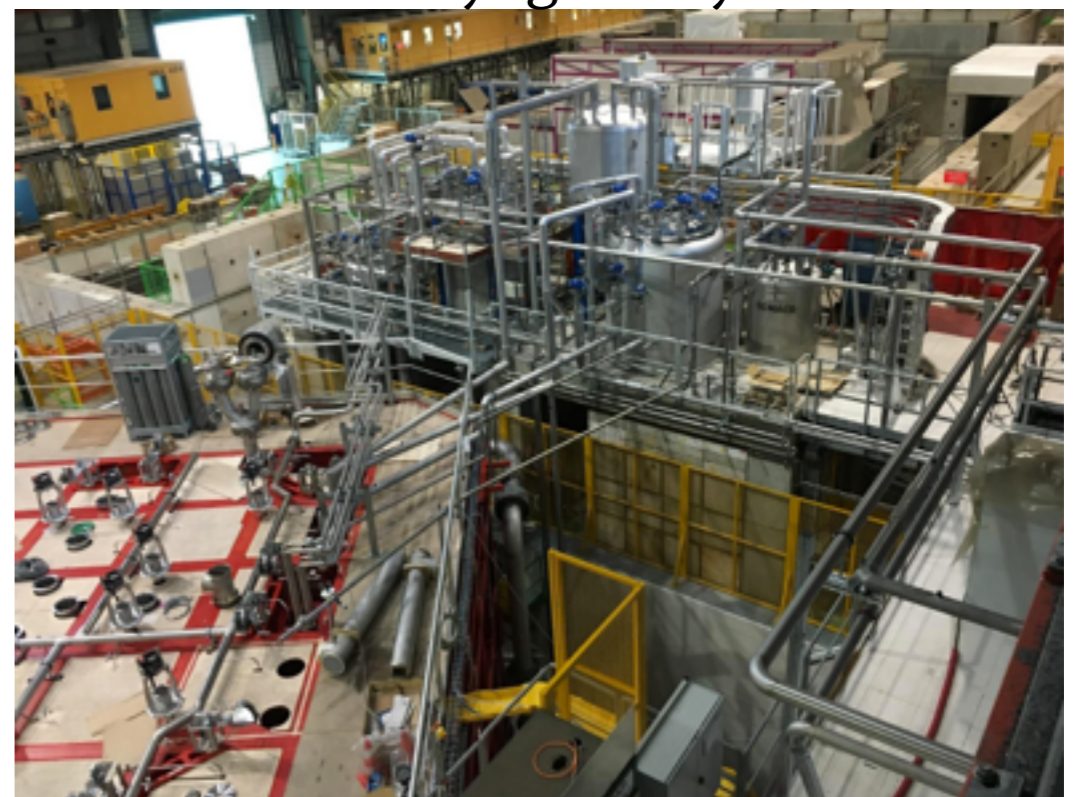
DP Cryogenic system
