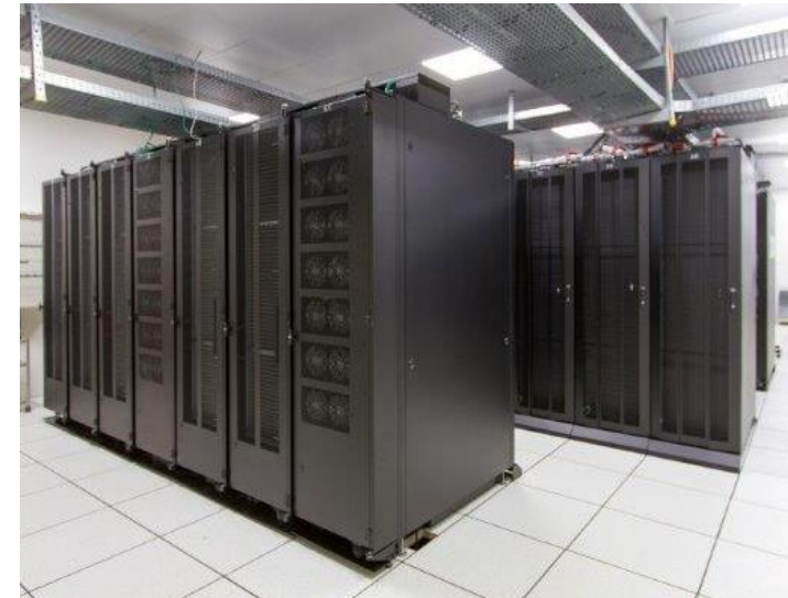
Data Center (aile 0) LHC Computing Grid - Tier2 Clusters HPC/GPU (all projects)
