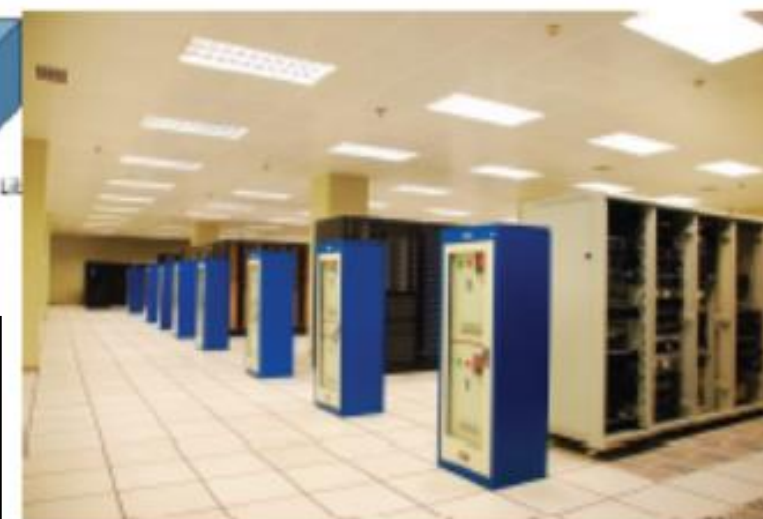
Power supply system
