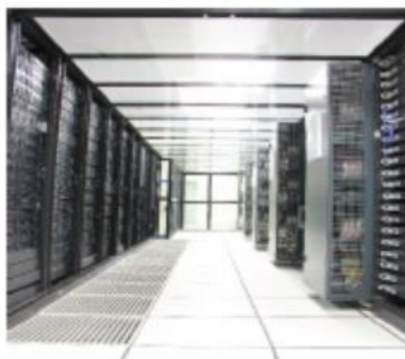
~18000 CPU cores Water cooling
