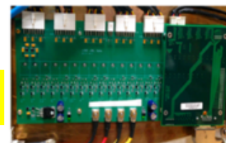
LVDB (low voltage)
