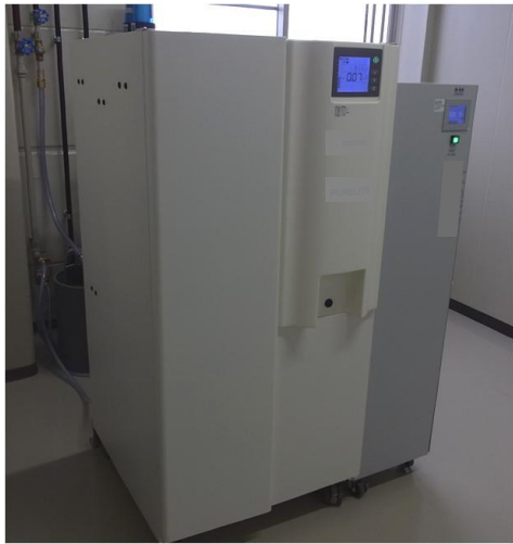
Ultra-pure water generator
