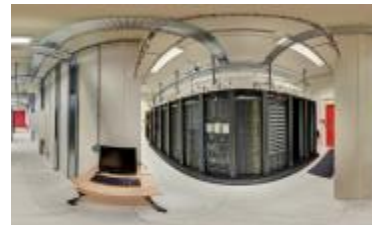
The Virtual Data computing room in Orsay after refurbishment
