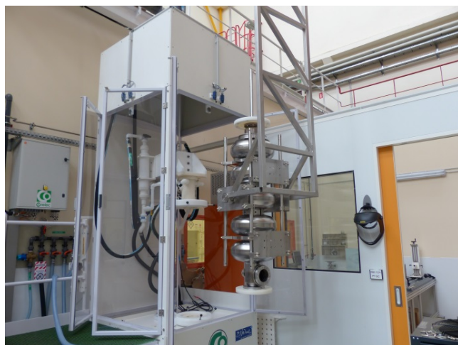
SPL Cavity insertion in the cabinet
