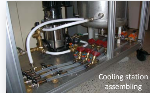
True scale leak less loop
