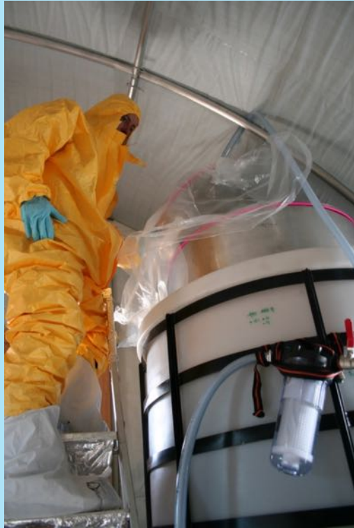
High efficiency double tank stainless steel smelter / 35kW propane boiler
